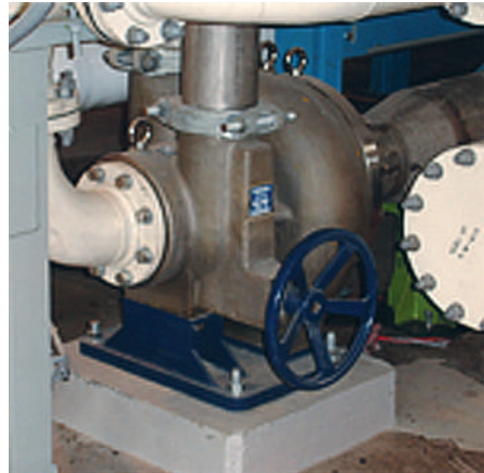
HPB-1000 in Jeddah, Saudi Arabia
