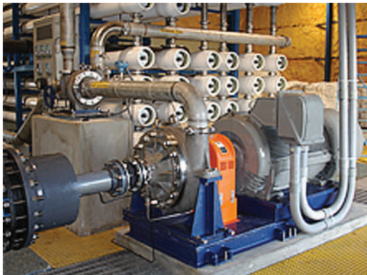
SSD-500 with HPB-5000 SWRO Facility
