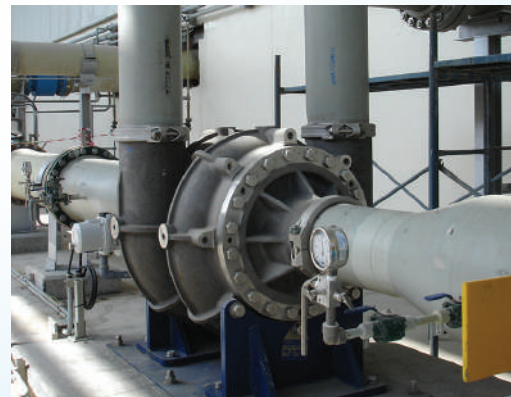
HPB-2800 installation SWRO - Saudi Arabia
